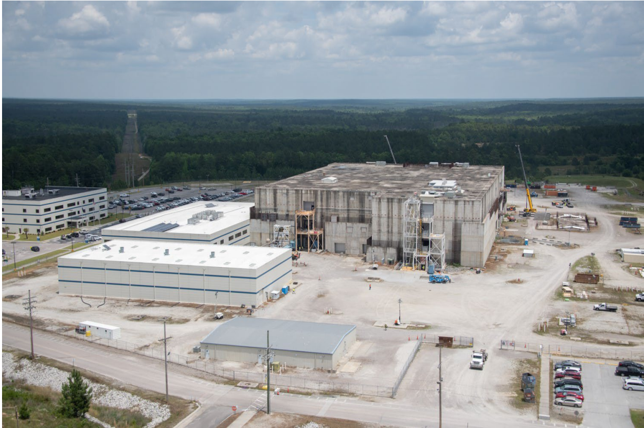
Aerial view of the SRPPF Main Process Building and supporting facilities
