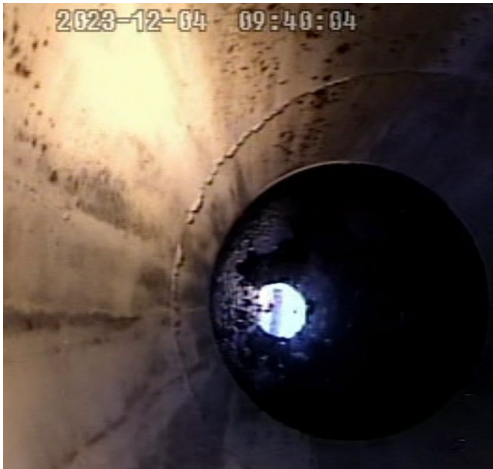
Cutline: This photo shows some of the welding material that was needed to be removed from inside a waste tank riser at the Savannah River Site. The material was ground away to allow for insertion of a mixing pump.
