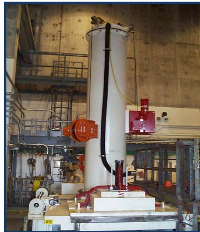
Shielded Transfer System (STS)
