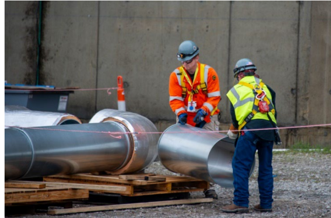
The installation of a temporary HVAC system for the Savannah River Plutonium Processing Facility (SRPPF) at the Savannah River Site (SRS) was completed in March. In this photo, workers transport air ducting in preparation for installation at SRPPF.
