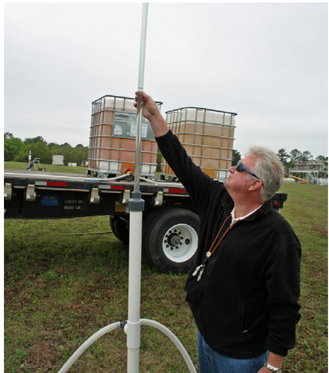
Savannah River Nuclear Solutions engineering and technical support specialist Keith Hyde measures the flow of vegetable oil during an injection process. The oil encourages growth of the underground population of naturally occurring, chemical-eating bacteria at the Savannah River Site
