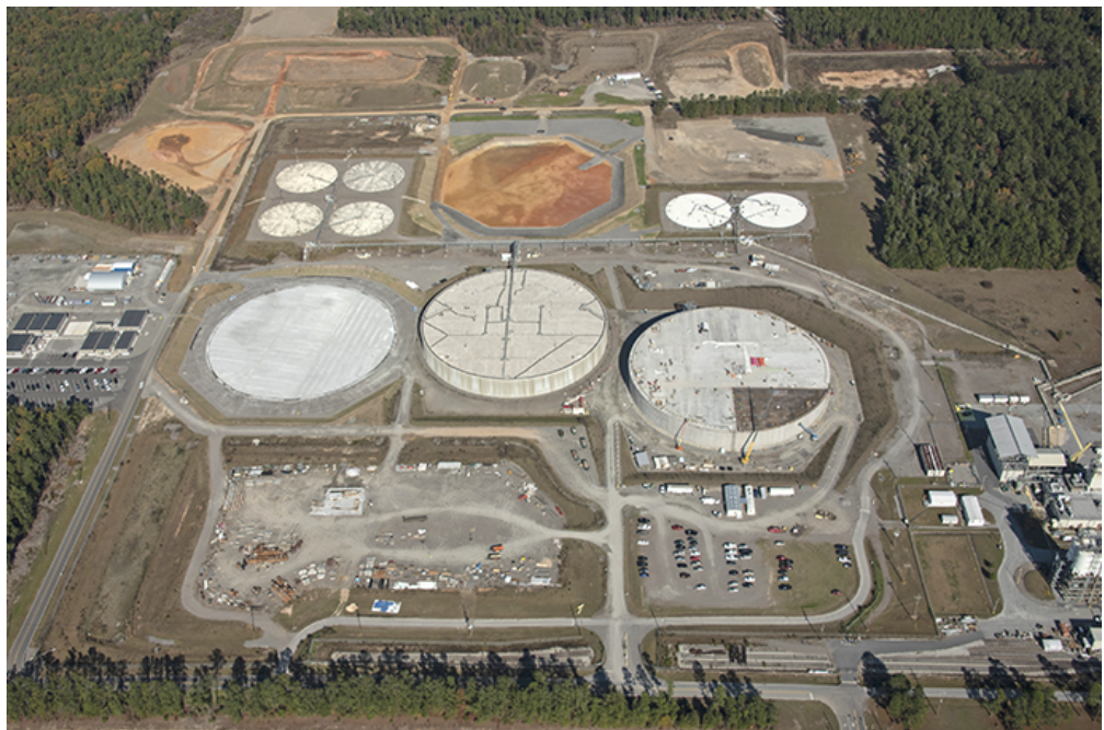
Workers build the roof of the mega-unit Saltstone Disposal Unit (SDU) 7, at right. Construction of the SDU 7's outer shell was completed Dec. 6. Also pictured are the construction sites for SDU 9, top, and SDU 8, left, along with the completed SDU 6, center.
