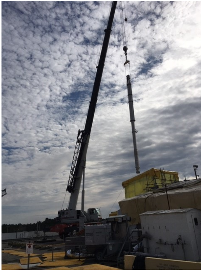
Workers use a crane to move a new pump to a Tank 41 riser for installation.
