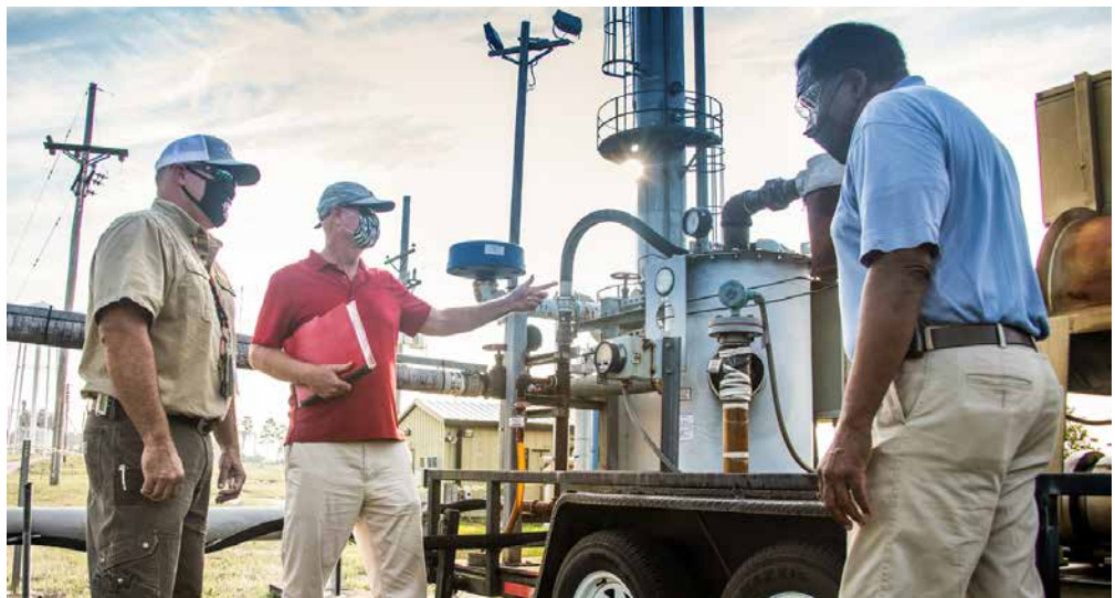
From left, Savannah River Nuclear Solutions mechanic Todd Cockrell, Engineer John Bradley and Project Manager Joao Cardoso-Neto plan the removal and dismantlement of a high-vacuum soil vapor extraction unit at the Savannah River Site.
