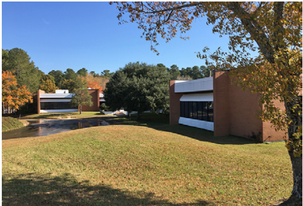
Crews recently replaced a deteriorating, leaking roof at the Savannah River Ecology Laboratory at the Savannah River Site.
