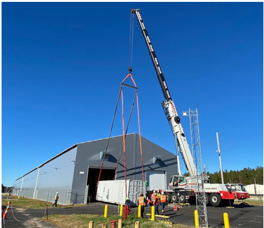
Crews move the Real Time Radiography unit into the covered Criticality Control Overpack pad for use in characterizing drums before shipment to a geological repository.
