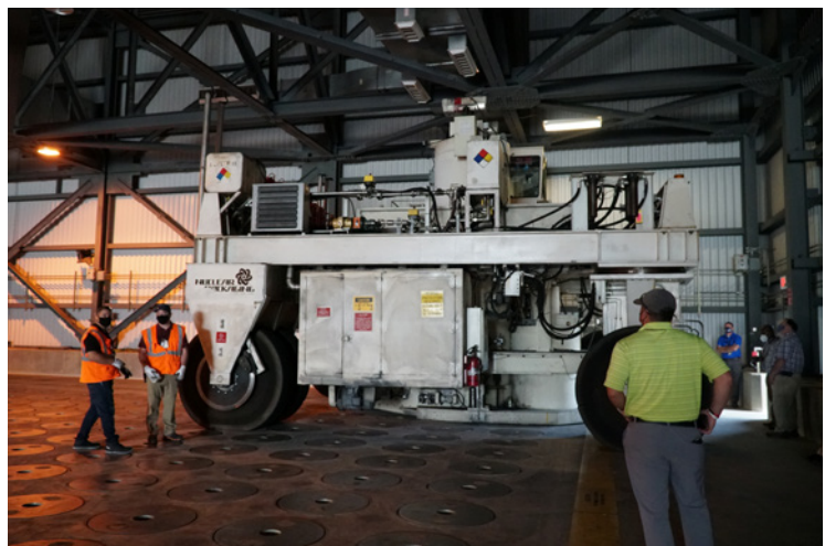
Crews at Savannah River Remediation successfully double-stacked the first canisters in an underground vault in the Glass Waste Storage Building 2 at the Savannah River Site using the shielded canister transporter.
