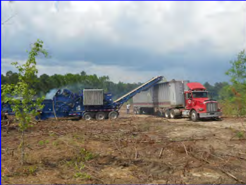
A grinder (left) sends logging debris piles thru a conveyor belt to a chip van.
