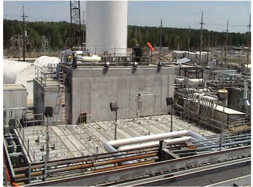
Modular Caustic Solvent Extraction Unit (MCU)
