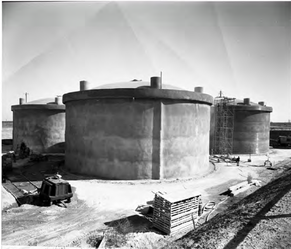
HTF Contains Four Type IV Tanks (Tanks 21, 22, 23, 24)
