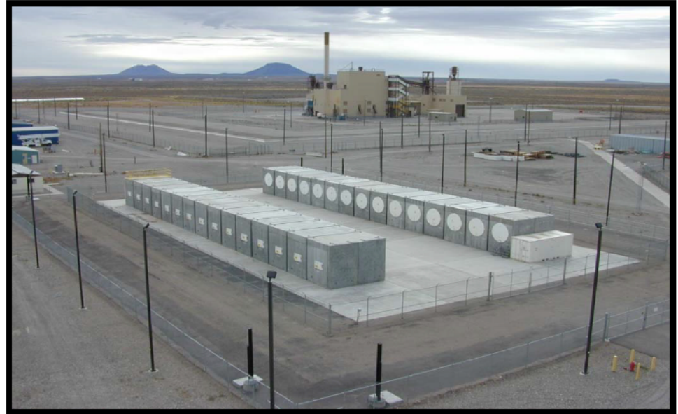
Three Mile Island ISFSI at Idaho National Laboratory
