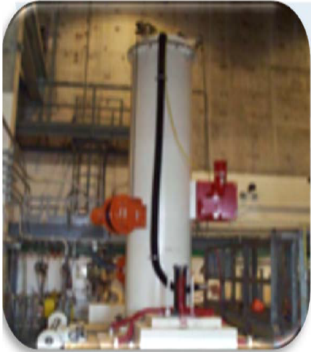
L-Basin Shielded Transfer System
