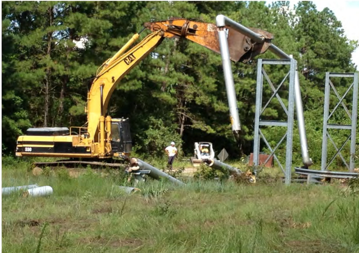
Abandoned Steam Lines
