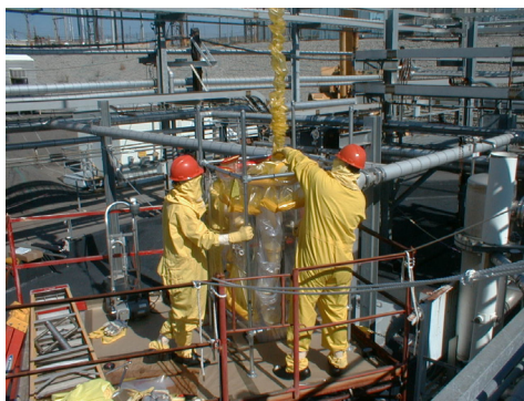
Employees conduct work at an SRS tank farm.
