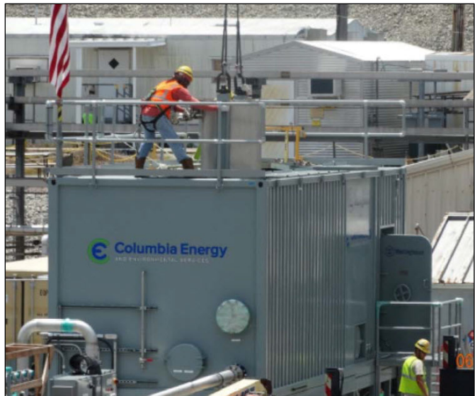
Ion Exchange Column Installed at TCCR
