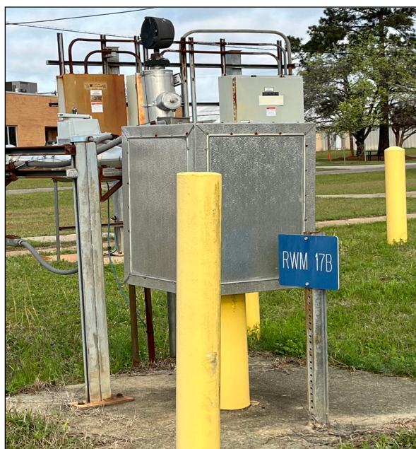
Recovery Well RWM 17B
